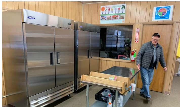
With new freezers in the background, facilities chair Glenn Rupp, completes instillation
